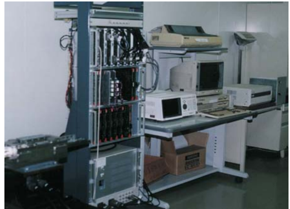
Fig. 5b Boards and Display of Control system
